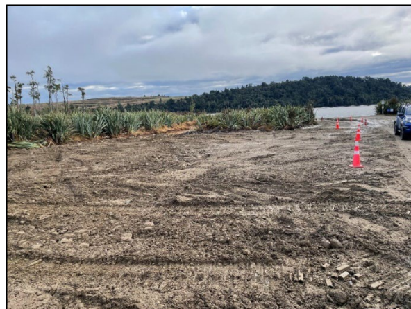
Figure 15: Vehicle Parking Area to improve safety and amenity for boat launching and trailer parking
