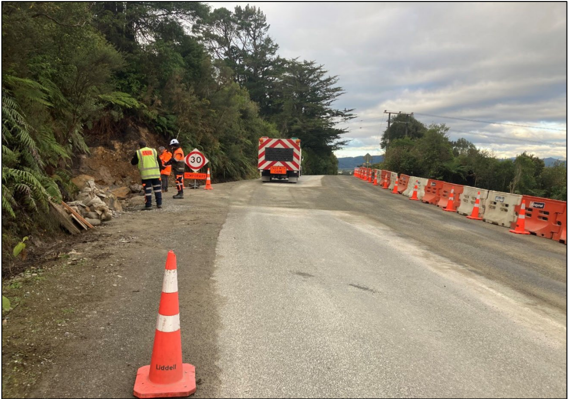
Figure 8: Taylorville Road Project – Temporary barriers in place, re-installation of safety barrier to be completed
