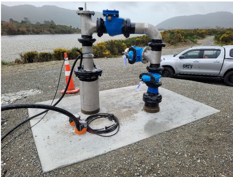
Fig 12: New bore #4 well head.
