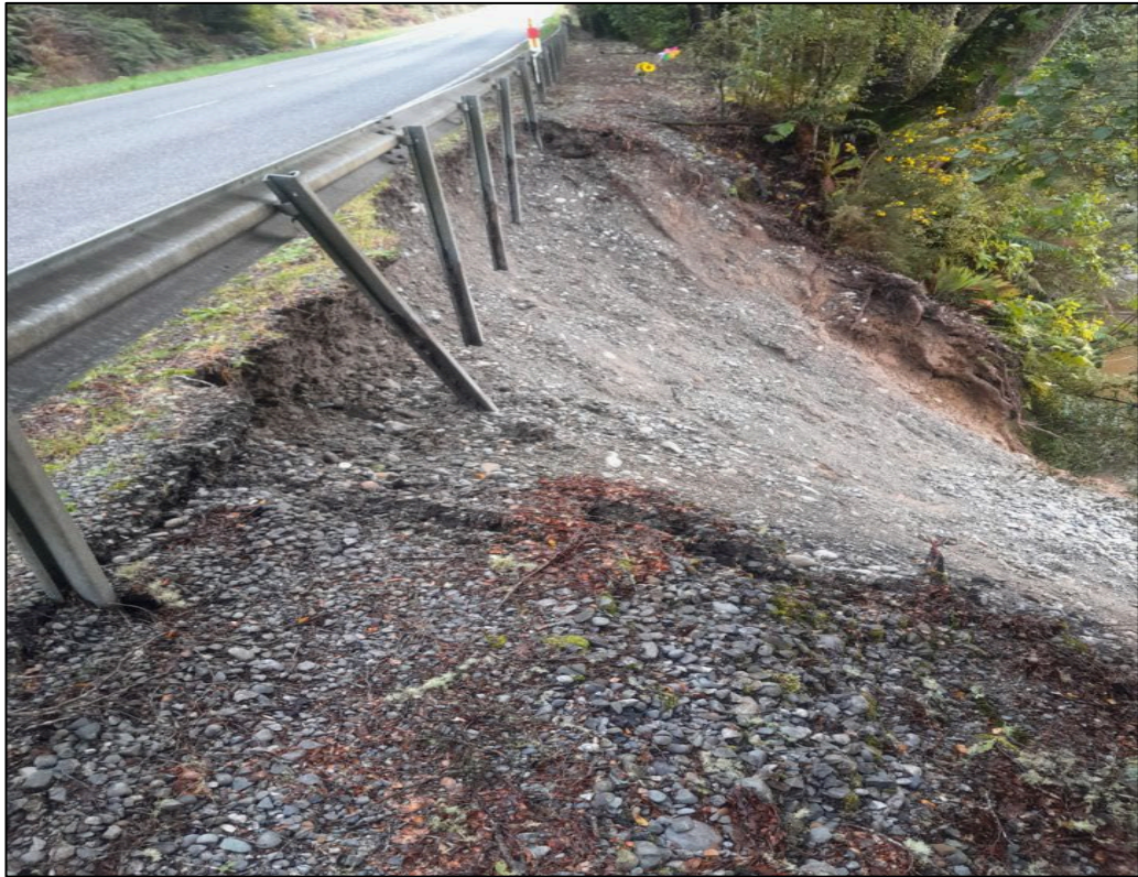
Fig 1: Slip on Taylorville- Blackball Road
