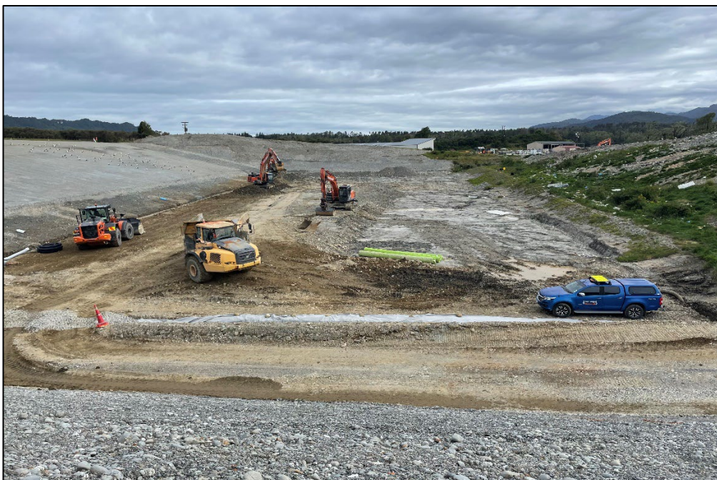
Figure 11: McLeans Pit Landfill looking east over new cell with drainage and mudstone excavation underway
