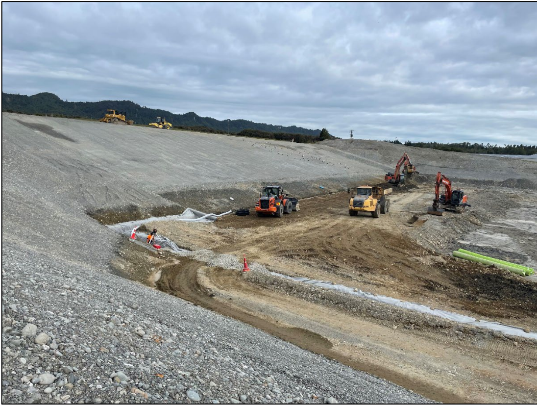
Figure 12: McLeans Pit Landfill Cell 3B Construction – looking southeast showing drainage is underway
