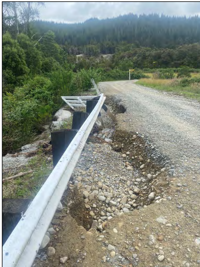
Fig 3: Damage sustained on Māori Creek Road, Greymouth
