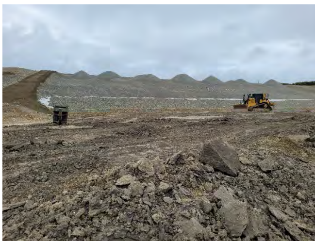
Fig 4: Construction continues on Landfill Cell3B – Photos showing the exposed mudstone layer, which the landfill is constructed within.
