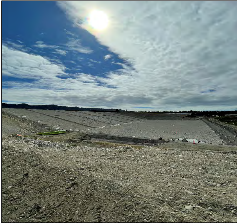
Fig 11: Photo showing current state of construction on new cell 3B – looking north.
