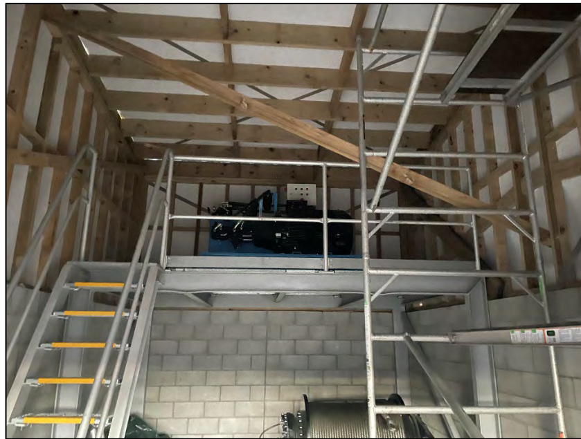
Figure 9: Internal Powerpack & Mezzanine with new winch below
