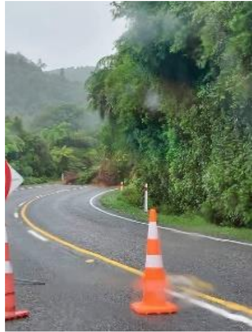
Photo 17. 24 Dec 2020 road closed by slip at Whitehorse Hill, just north of Fox River, left. Photo: NZTA
