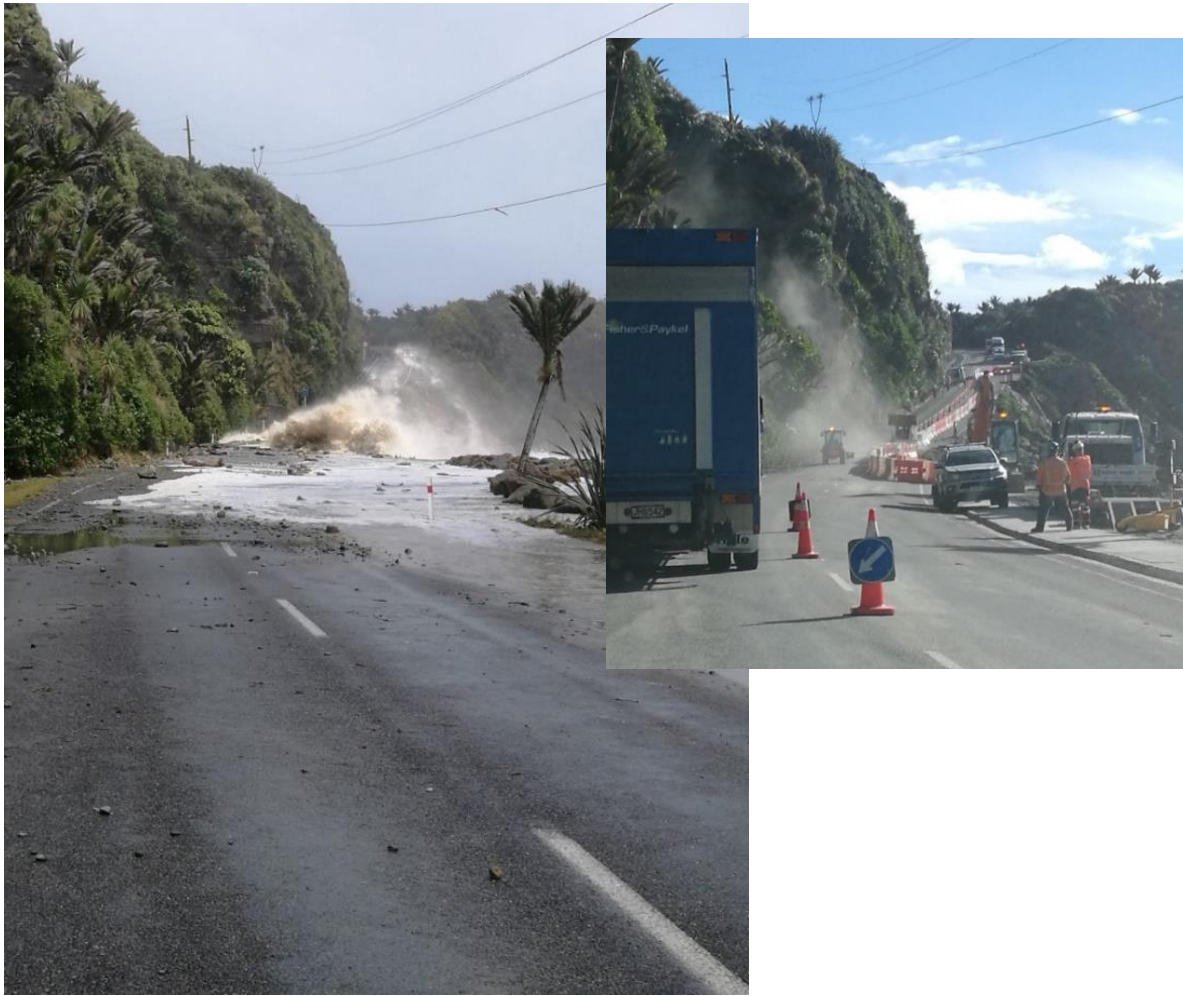
Photo 14. 01 February 2018, just north of Dolomite Point during ex-Cyclone Fehi, photo left. Photo 15. Repairs begin, photo right. Both show SH6 demolished almost to the centre line.
