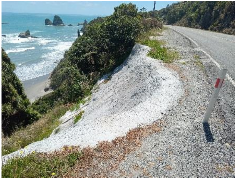
Photo 24. A costly 2023 repair to the road edge just north of Waianiwaniwa/ Ten Mile. Note the remaining narrow shoulder beside a steep drop, leaving a pedestrian, cyclist or motorist nowhere to go if needing to avoid an oncoming or overtaking vehicle.
